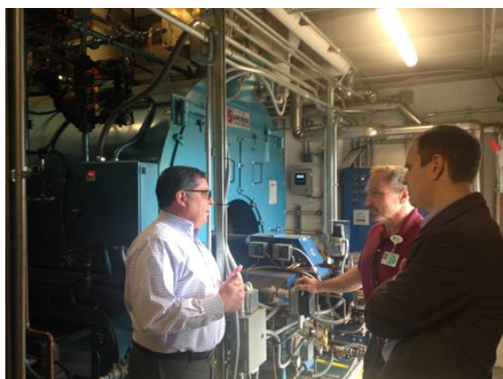
The main behavioral goal of the program was for frontline facilities management staff to review and maintain set-point adjustments in their Building Automation Systems
